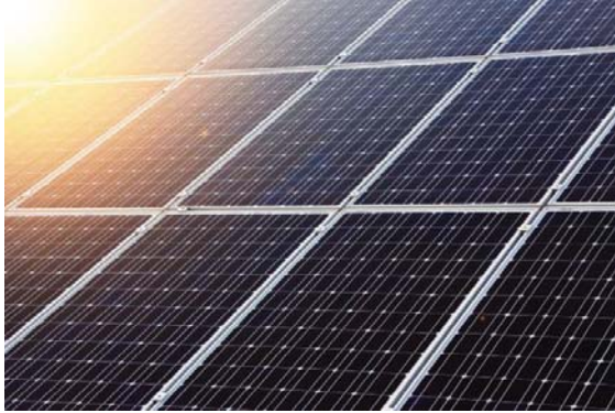
Figure 18 Solar panels source: aardvast.nl
