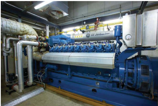
Figure 16 Cogeneration installation source: lekhabo.nl
