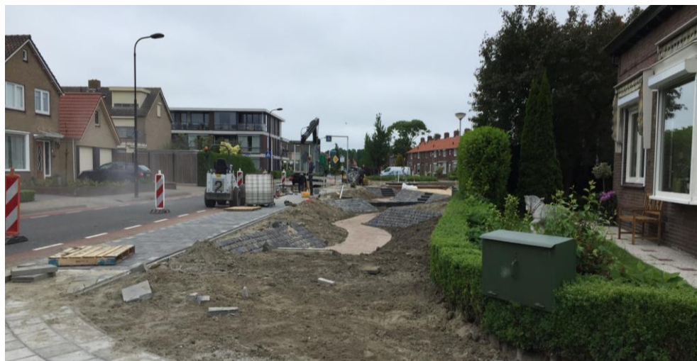
Figure 9 The wadi is currently under construction (May 2017) (picture taken during location visit)
